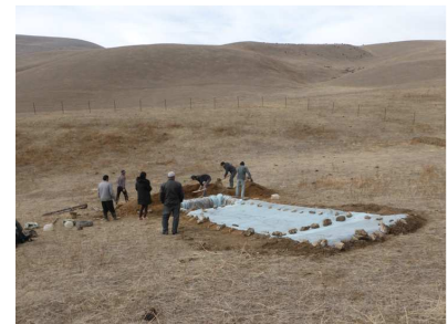
Stones are used to stabilize the rainwater collection area against strong winds
