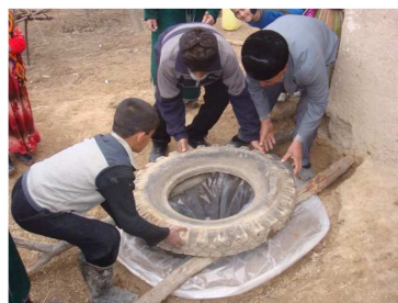
Placement of a car tire at the top of a water storage pond through which water in- and outtake are achieved
