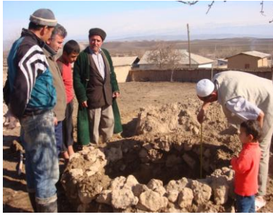
Confirming again the exact dimension of the rainwater harvesting structure under construction
